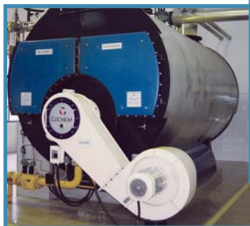
The Shanghai facility's new natural gas boiler.
